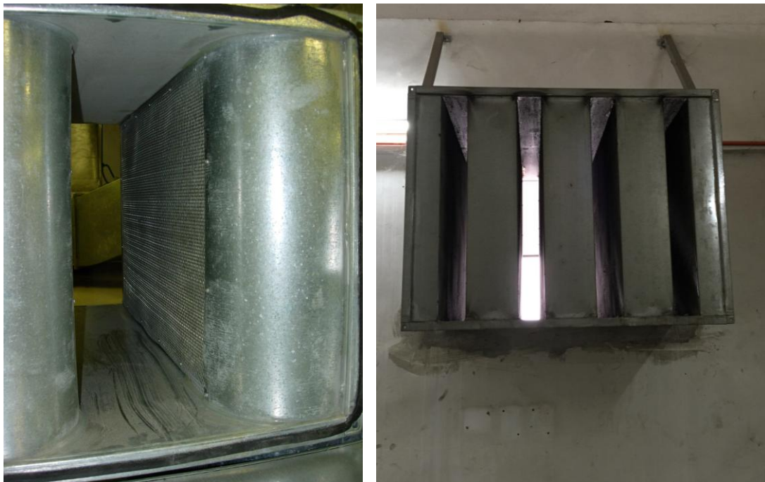
Figure E-20: Dissipative silencers in a plantroom application, with a close up view of typical sound absorption splitters
