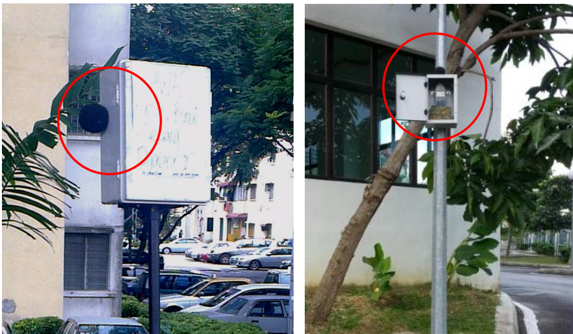
Figure B-15: Examples of unacceptable use of sound level meter installed in a casing as an alternative to permanent noise monitoring units
