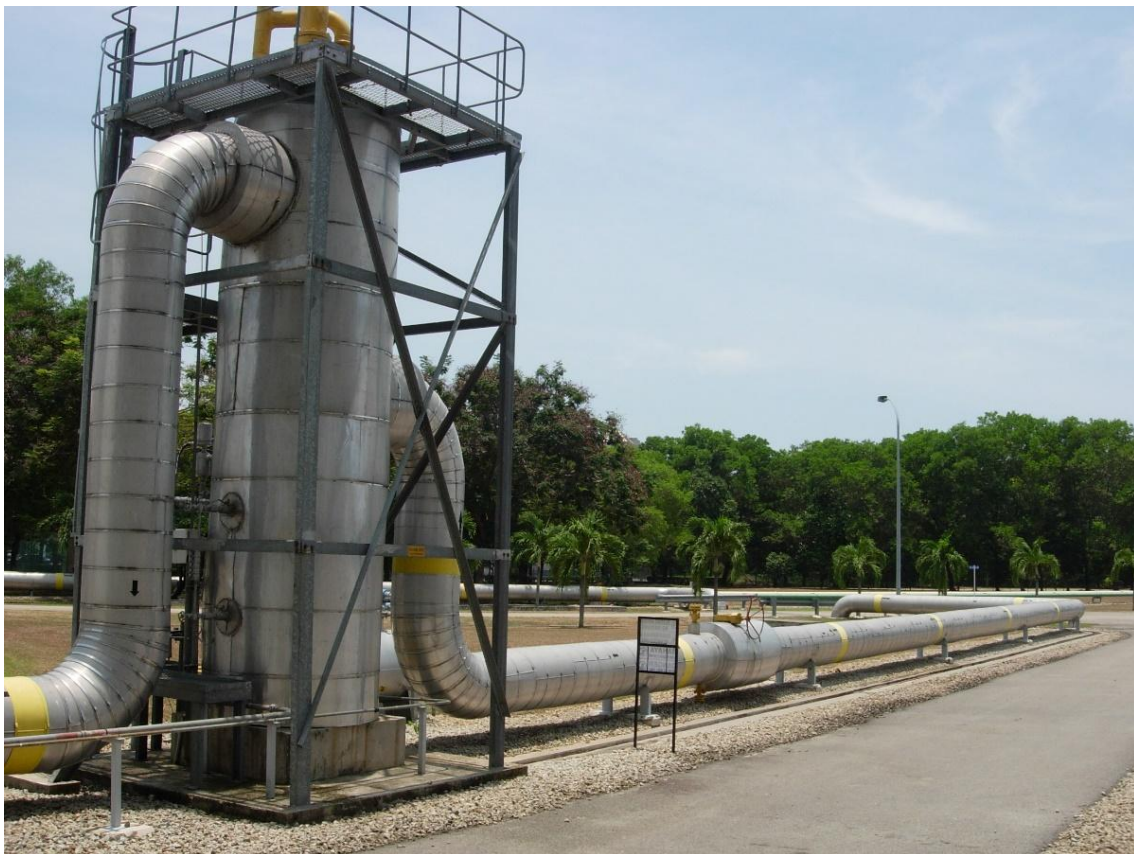
Figure E-26: Example of gas pipes external lagging in industrial noise mitigation
