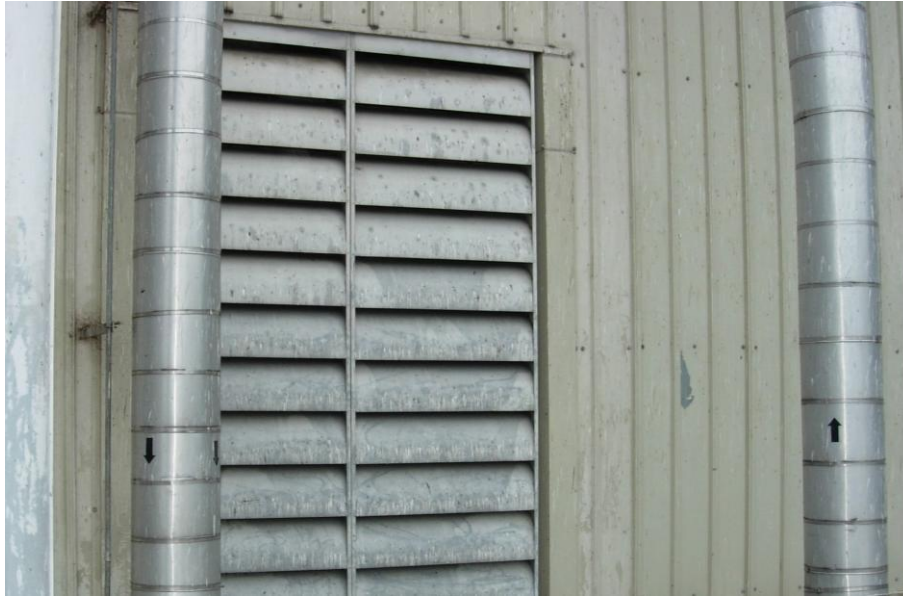
Figure E-22: Acoustic louvers used for natural ventilation opening in power station turbine hall
