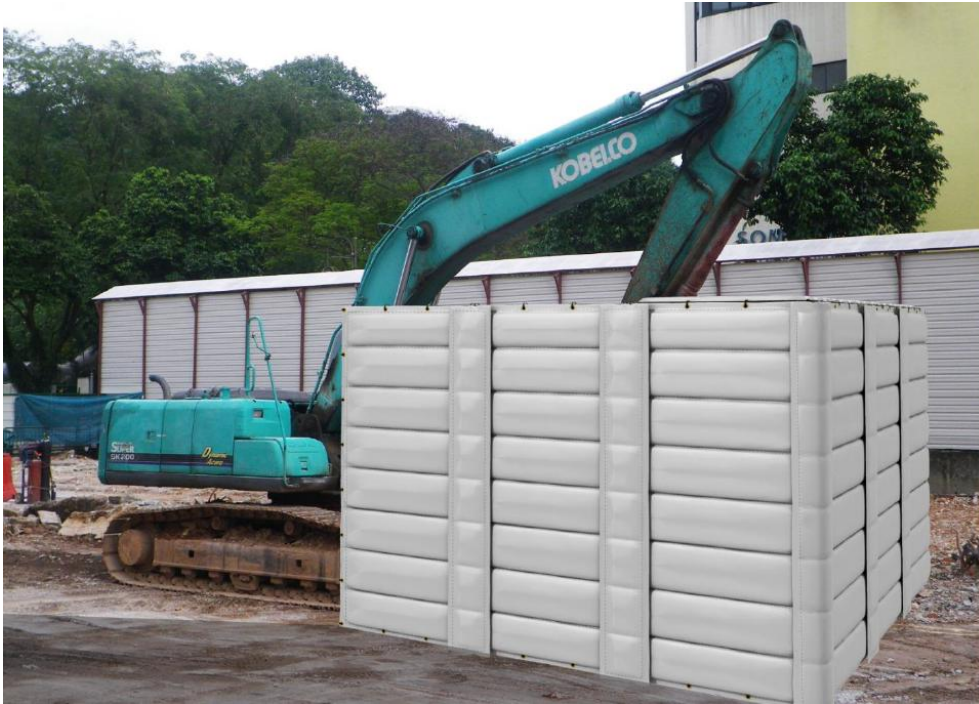
Figure E-11: Movable barriers used for mobile noise source in construction works
